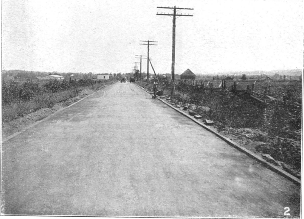
Montreal-Quebec highway. Making asphaltic concrete in 1919, at L'Ancienne-Lorette.— 1. Plant of the contractors, Laganière, Houde & Co.—2. Foundation layer in macadam ready for receiving the asphaltic concrete.
