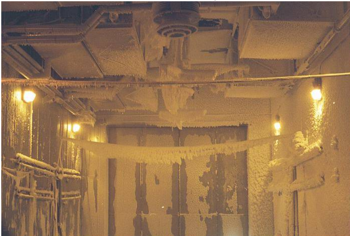
Photo 6.4 Accumulated Snow Following Test
