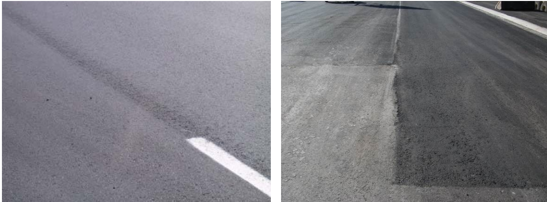
Figure 4-5: Examples of Poorly Constructed Joints
