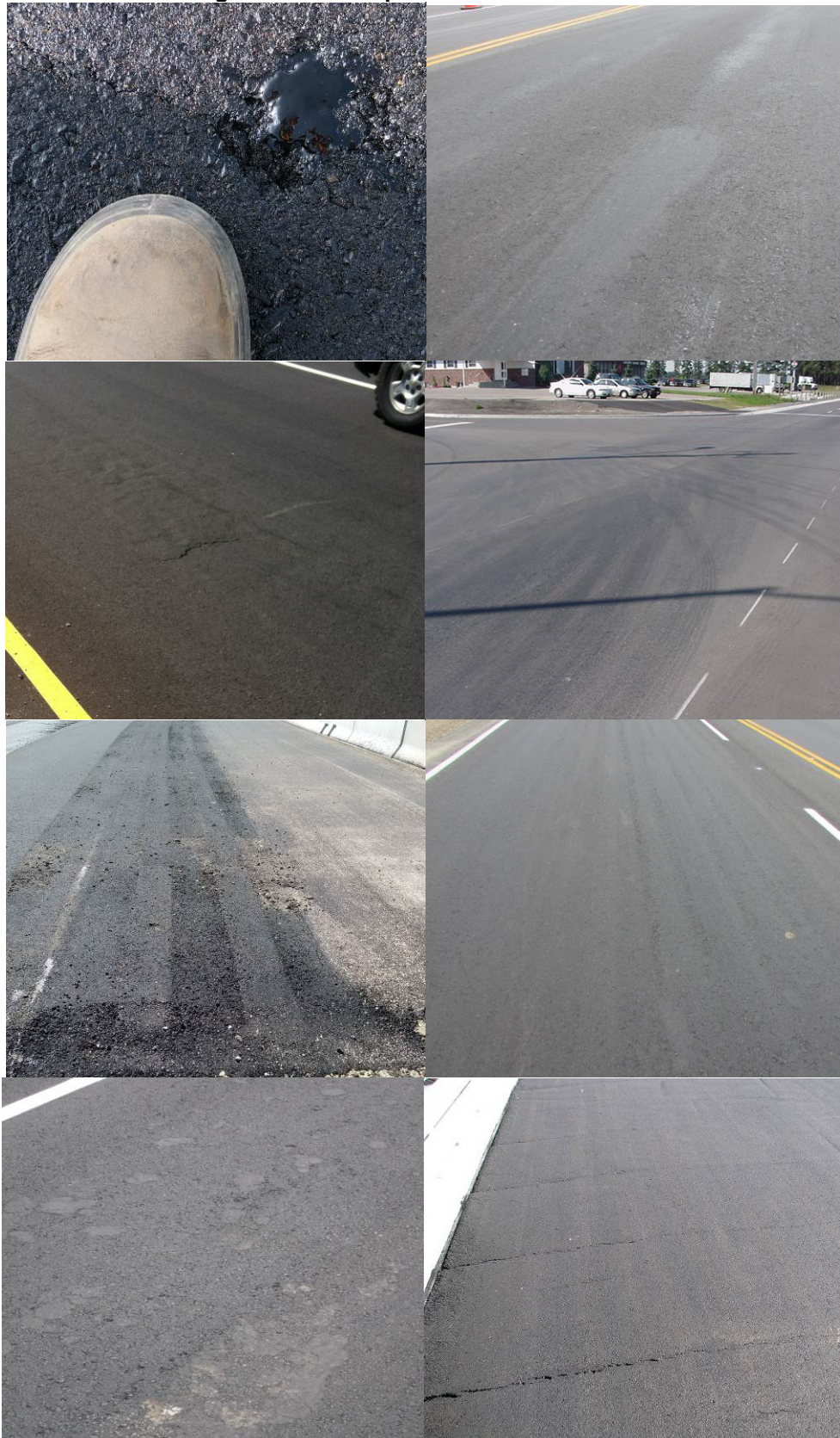
Figure 4-2: Examples of Surface Defects
