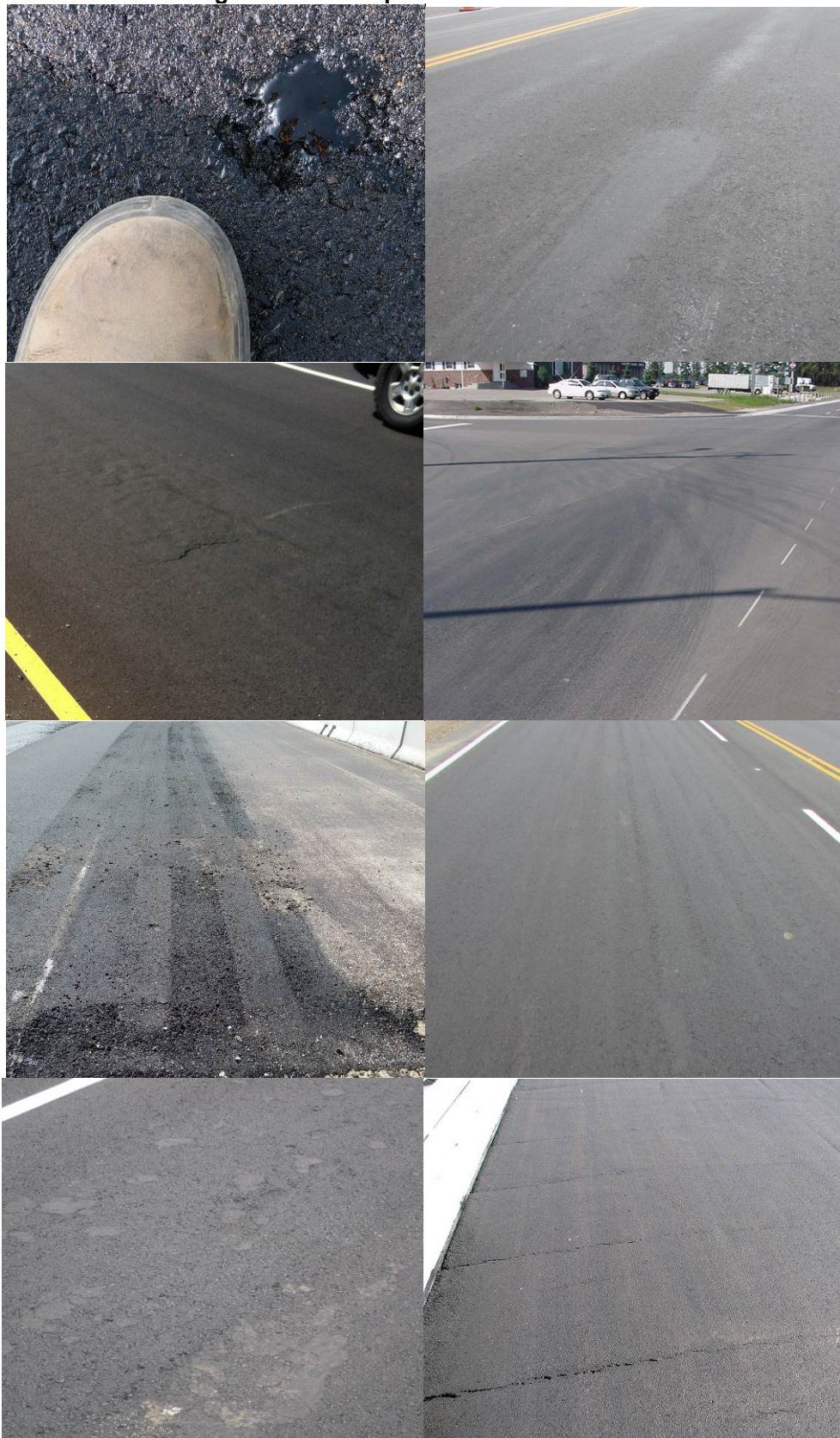
Figure 4-2: Examples of Surface Defects
