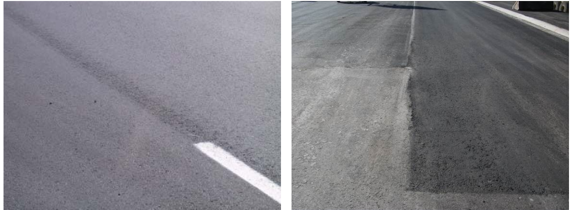
Figure 4-5: Examples of Poorly Constructed Joints
