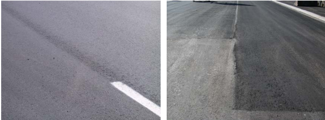
Figure 4-4: Examples of Poorly Constructed Joints
