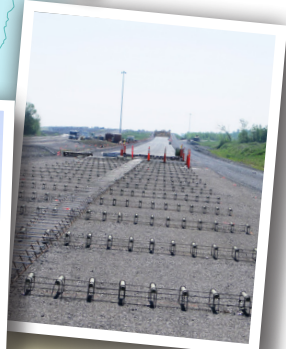
Concrete slabs for Autoroute 30 between Rue Saint-François-Xavier and Autoroute 15. The Eastern section of Autoroute 30 will be paved entirely in concrete.
