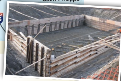
Construction of a footing for the westbound Autoroute 30 overpass over Chemin Candiac.
