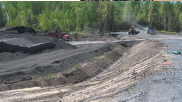
An impressive quantity of materials was used to consolidate the sector's subgrade.
