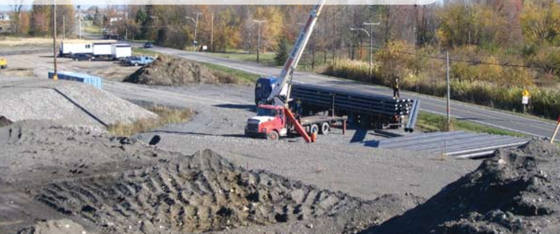
Work at the site resumed in October following completion of the consolidation of clay soils.
