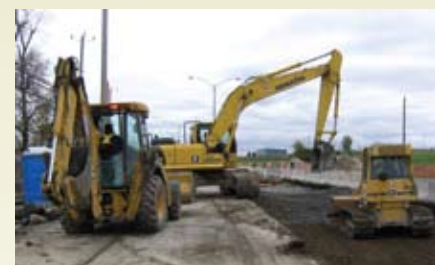
The work to relocate route 236 in Beauharnois was also carried out in the fall.
