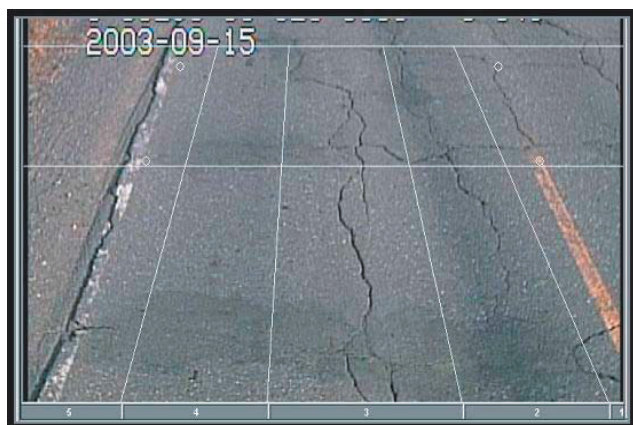
Figure 3: Analyse de la fissuration
