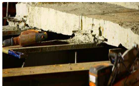
Figure 6.26 Section G-G – Béton sain
