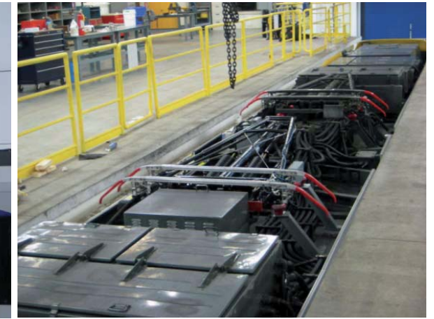
Roof top (pantographs lowered)
