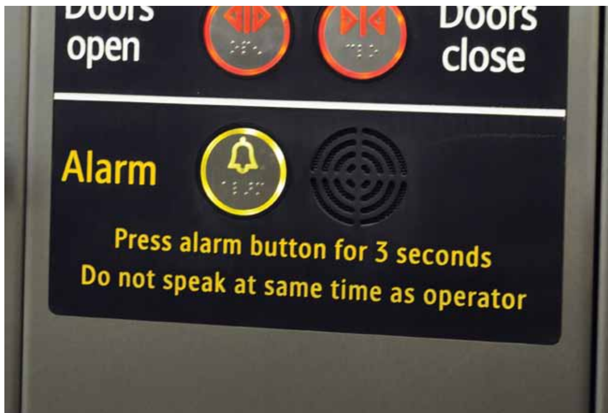
Figure R2.1 Lift controls, showing the alarm button
