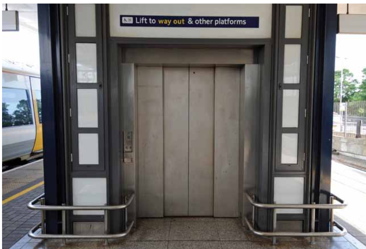
Figure R1.1 A typical station lift
