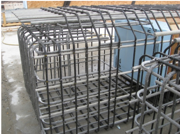
Fig. 3. CFRP stirrups in girders – MTO NW region
