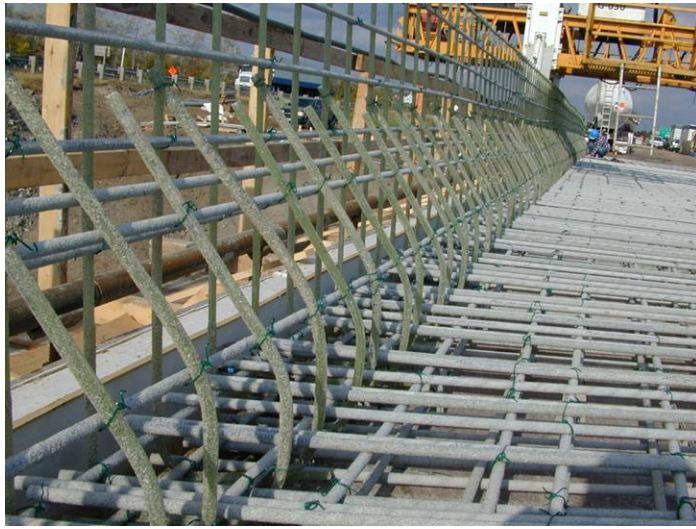
Fig. 5. Top & bottom FRP in decks and barriers – Quebec 2004
