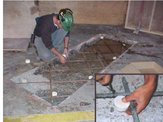
Figure 2: Alkali-Activated Discrete Galvanic Anode Installed For Localized Protection Around Concrete Patch Repair
