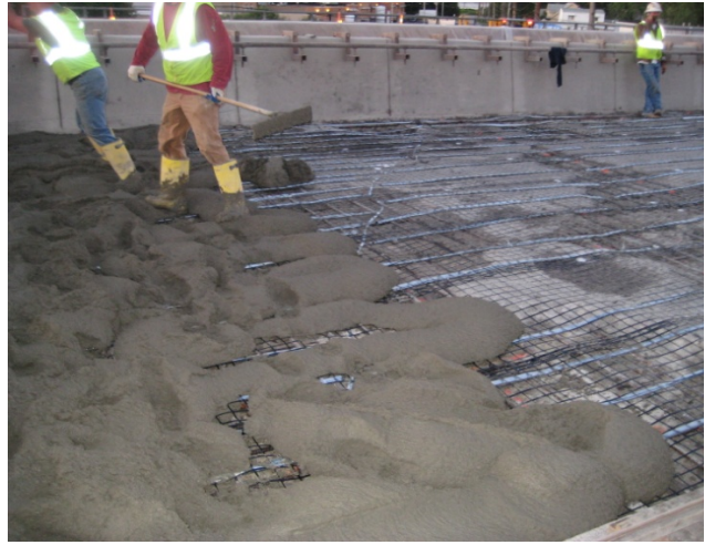
Figure 10: Concrete Overlay Placement over Distributed Galvanic Anodes on Ohio DOT Bridge Deck
