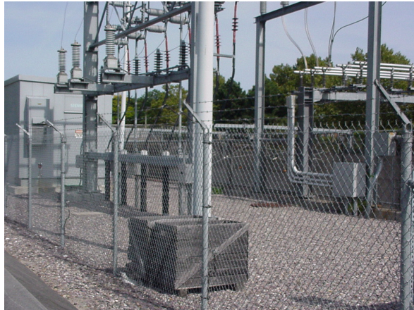
Figure 21 Typical 2x25 KV System Autotransformer Station
