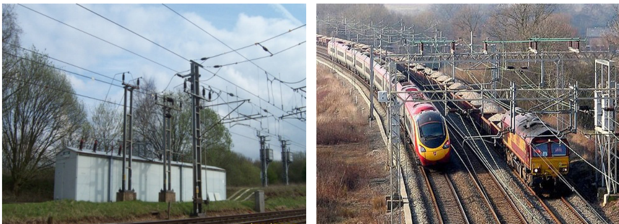
Figure 19 Typical Overhead Contact Systems
