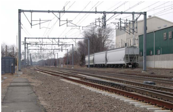
Figure 8: Typical Multi-Track 2x25 KV OCS and Feeder System with Side Portal Construction
