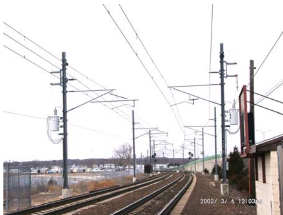
Figure 7: Typical Two-Track 2x25 KV OCS and Feeder System with Side Pole Construction
