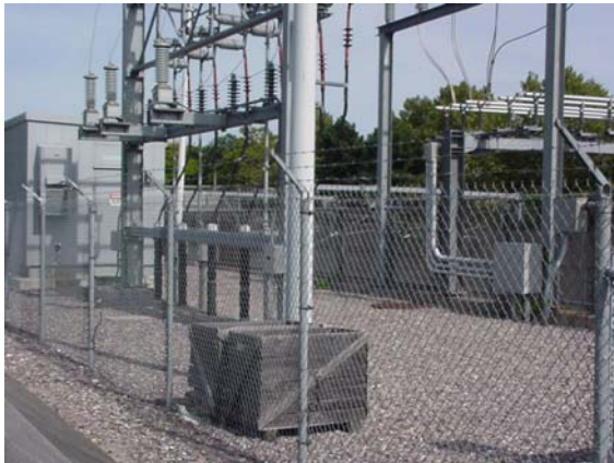
Figure 10: Typical 2x25 KV System Autotransformer Station
