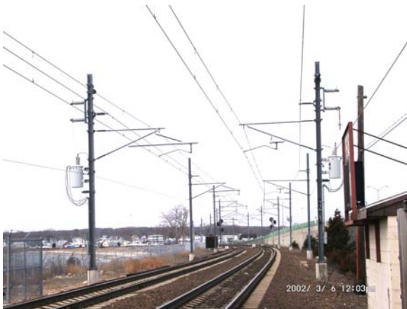
Figure 2-4 – Typical Two-Track 2x25 kV OCS and Feeder System with Side Pole Construction
