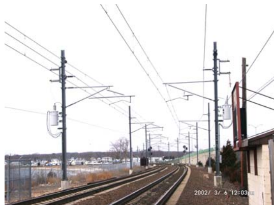
Figure 12: Typical Two-Track 2x25 kV OCS and Feeder System with Side Pole Construction
