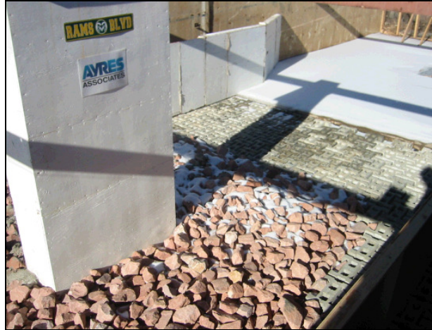
Figure 12.12. Loose riprap, ACB, and contraction wall installation (note loose riprap on the near side of the pier and partially grouted riprap on the far side).
