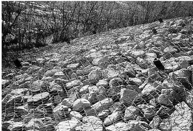
Figure 6.2. Wire enclosed riprap used for guide bank side slope protection at I-25 crossing of Rio Galisteo, New Mexico (NMSHTD).
