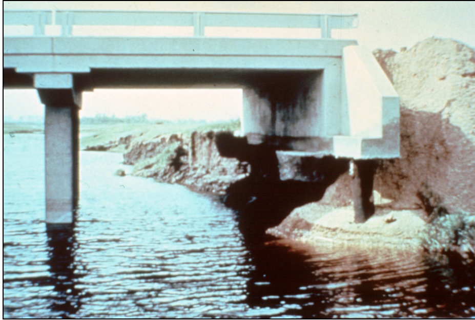
Figure 14.1. Scour of bridge abutment and approach embankment.
