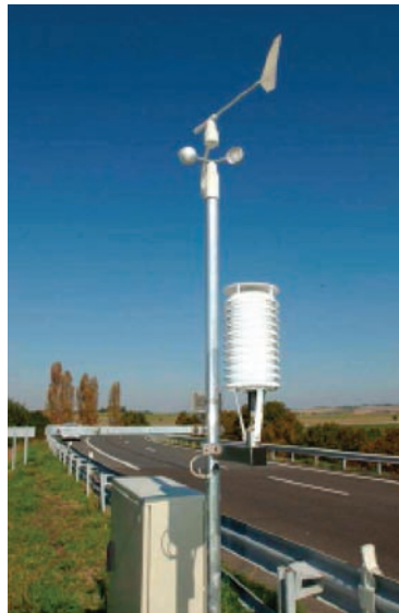
Road weather information system.
