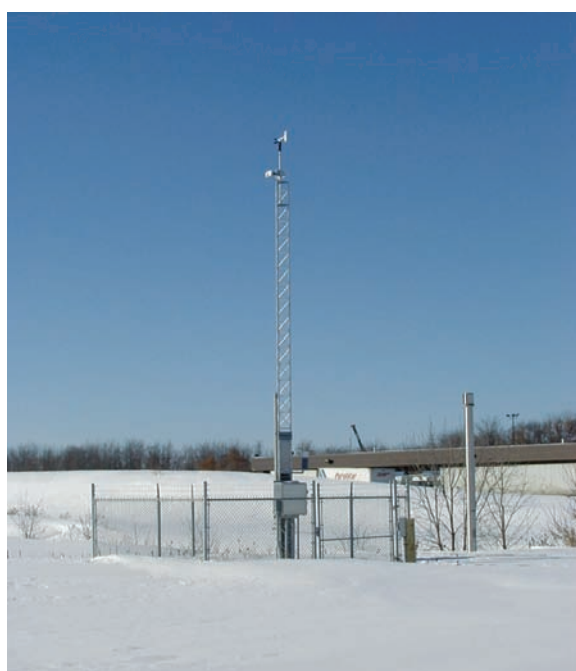
Typical Canadian RWIS installation
