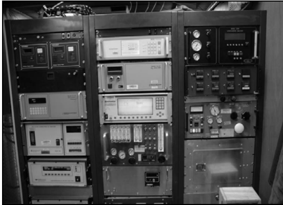
Figure 10a: Emission Equipment
