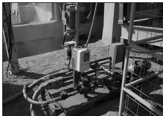
Figure 7b: Pump/Metering System
