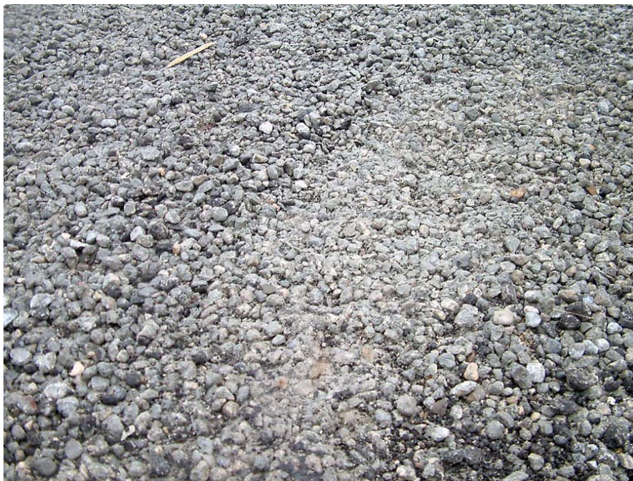
Figure 8. Areas of Severe Raveling
